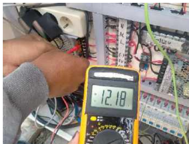
Gambar 3. 19 Pengukuran Tegangan Output Power Supply 12V
